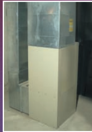
Hydro-air and heat pump backup
