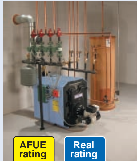
Typical high-mass boiler with indirect water heater.
